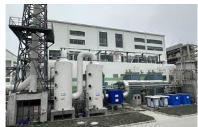
Environmental response by waste gas treatment scrubbers and MBR water treatment facilities
