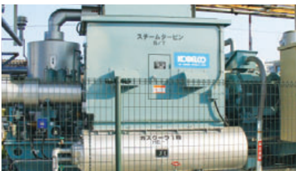
Steam turbine compressor (Shizuoka Plant)
