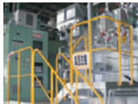
Boiler converted to utility gas (Amagasaki Plant)
