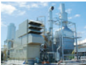
Cogeneration system (Shizuoka Plant)
