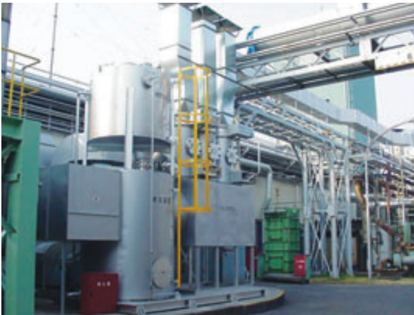
Exhaust gas treatment facilities
