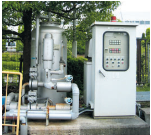
Rainwater treatment equipment (Nara Plant)
