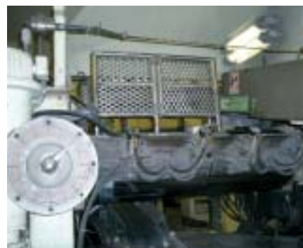
Safety fence installed to prevent potential danger from contact with a roller (Utsunomiya Plant)
