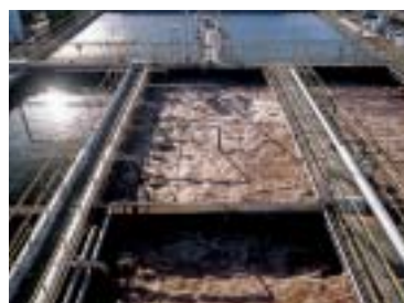
Activated sludge treatment equipment (Shizuoka Plant)
