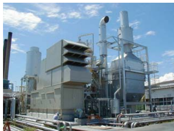
Co-generation system (Shizuoka Plant)
