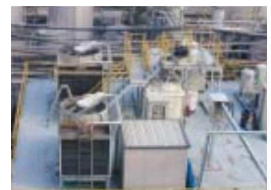
Water recirculation equipment (Amagasaki Plant)
